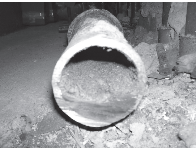
Cross-section view of original 42-year-old plumbing pipes at the High School currently contain significant blockage due to decades of built-up sediment deposits.
